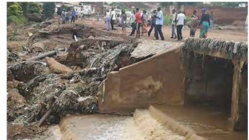
Photo: Flash flood damages in Lilongwe, Malawi, January 2019. Department of Disaster Management Affairs, Malawi.
