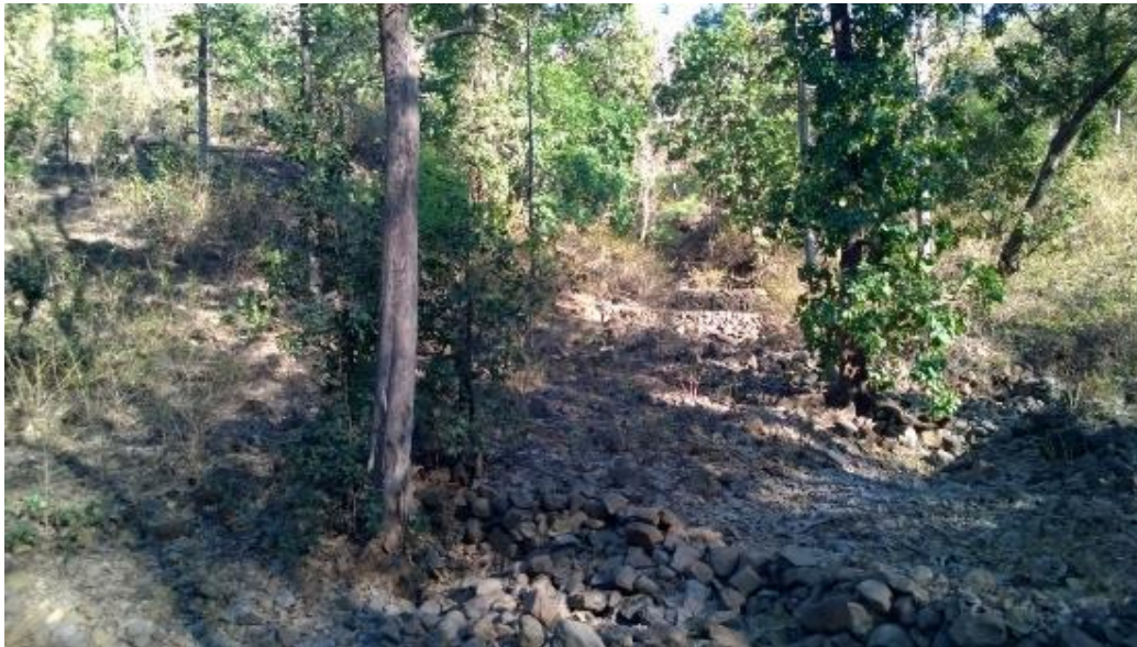
Picture 9 – Loose boulder check dams in series in Parasda village, Bhaura range, Betul
