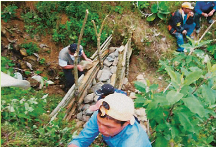
Implementing erosion control measures resulting from land use planning in Guatemala (see A2)
